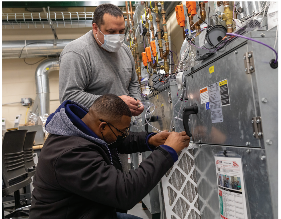
Students at Milwaukee Area Technical College, which uses BEST's curriculum, install a pressure switch to determine if an air filter is dirty.
