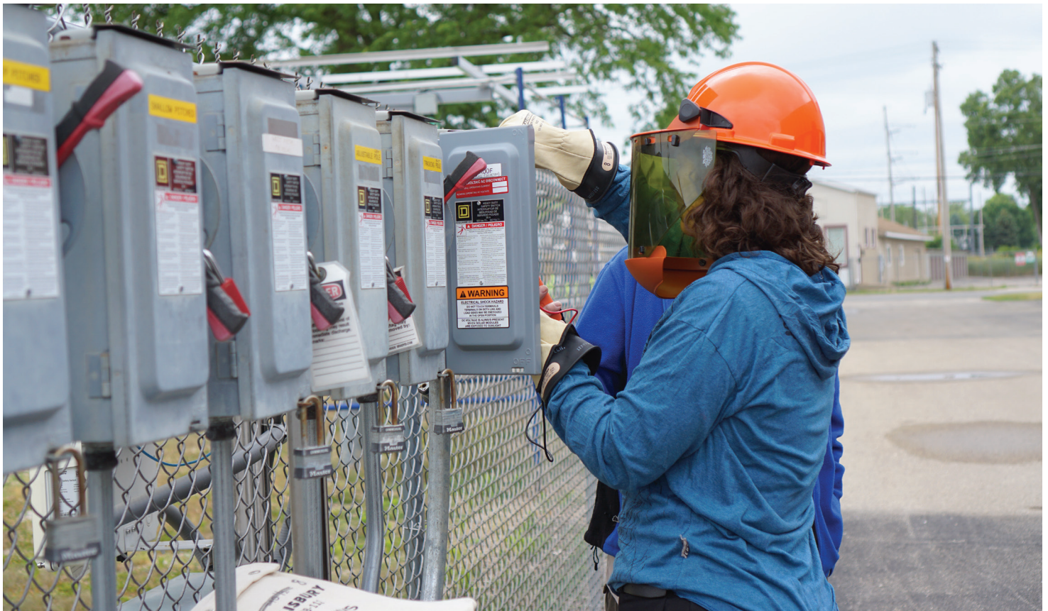
A student measures the electric potential across a solar photovoltaic disconnect switch, a maintenance task taught in CREATE's curriculum.
