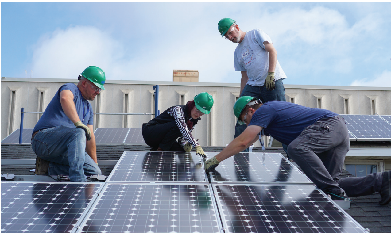
Participants put the finishing touches on a solar energy installation during a Center for Renewable Energy Advanced Technological Education's (CREATE) Faculty Energy Institute. (See page 30)
