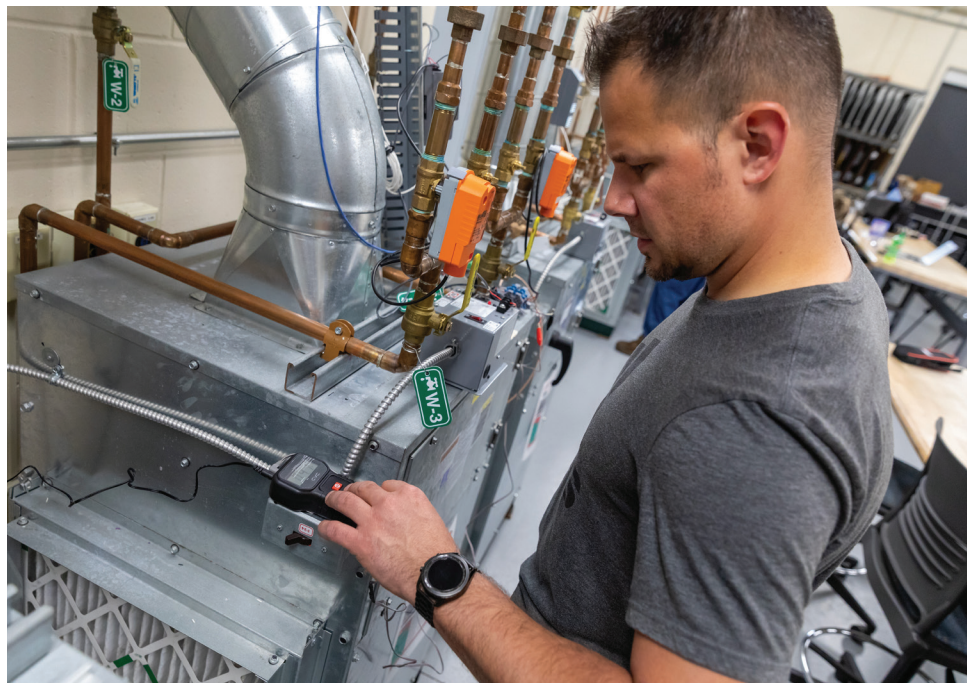
ACABT teaches students a wide array of skills, including how to check control signals to verify a motor's operating speed.
