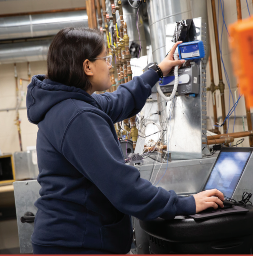
A facilities maintenance apprentice troubleshoots a building automation controller by using a Bluetooth connection device at Milwaukee Area Technical College, a BEST partner.
