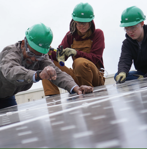
Students install solar panels on the pitched roof that is part of the outdoor lab at Madison Area Technical College.
