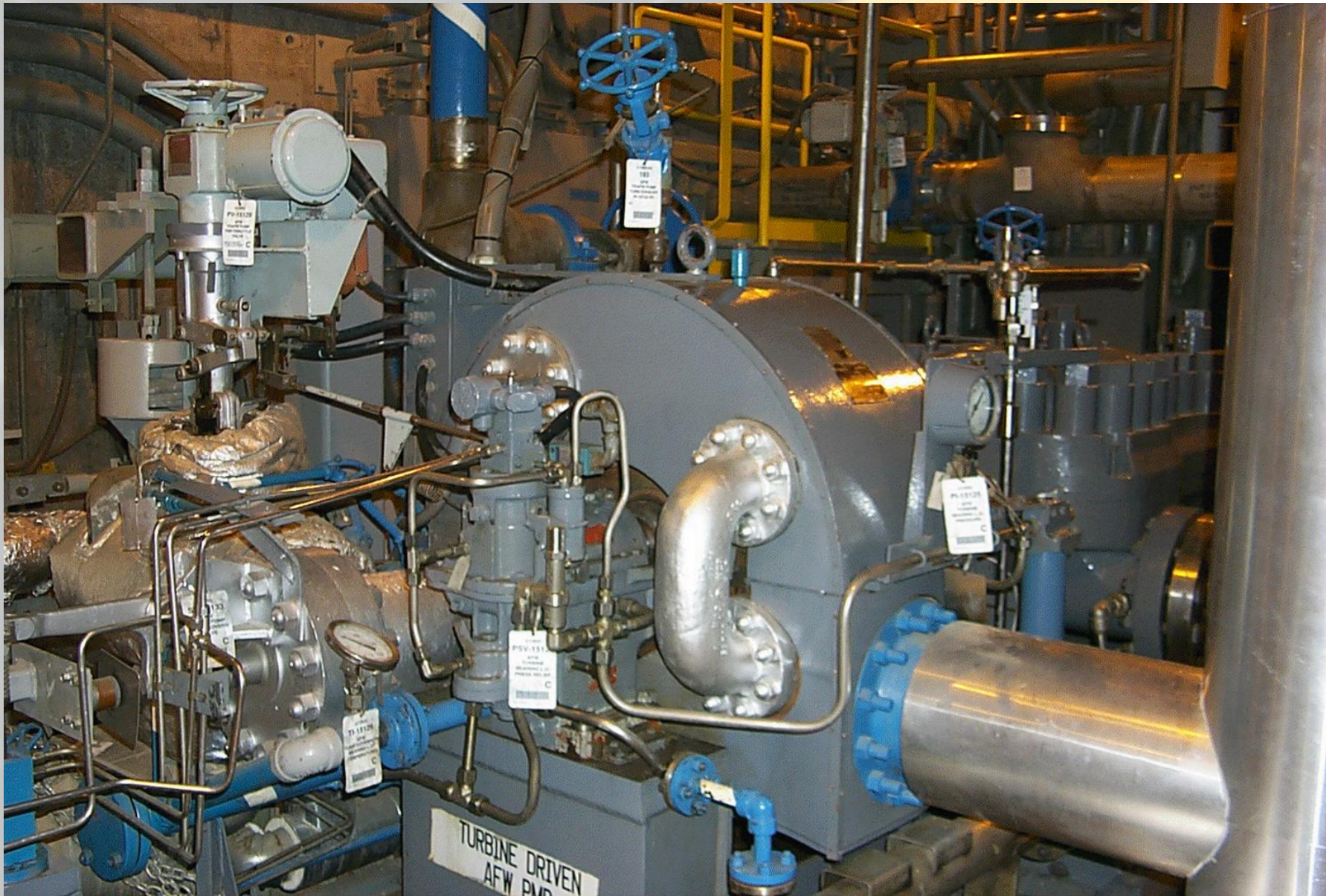
Turbine Driven AFW Pump
