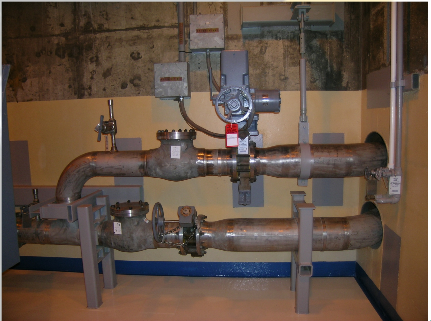
Motor Driven AFW Pump Suction Piping
